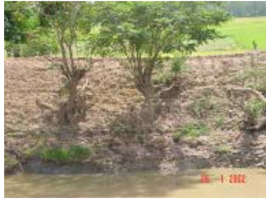
Trees are not effective against flood erosion, note the exposed roots
