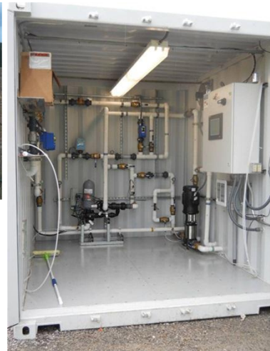
Pre-treatment and Distribution System. The engineered pre-treatment and distribution system automatically adjusts to changes in leachate production, leachate quality, and weather conditions to ensure proper operation.
