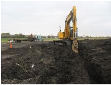
Underground Piping. Force mains are installed to convey leachate to the vetiver planting area.
