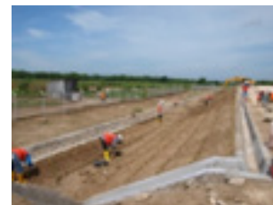
Support David J Booth in supply and plant vetiver system at East Java, Exxon Mobil
