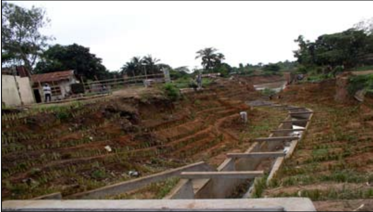
Photo 7: Gully and drainage channel with recently planted vetiver protection.
