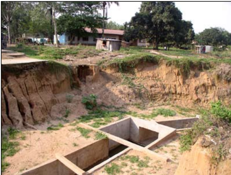
Photo 6: Badly eroding gully and unprotected drainage. Most civil engineering work to stop the progression of this
