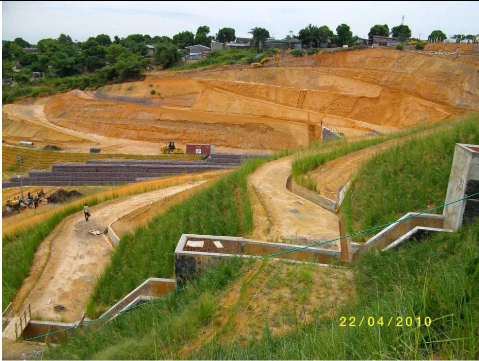
5. Construction of drain, terramesh retaining wall and the planting of vetiver grass
