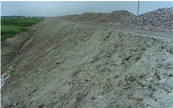
Railway embankment subject to serious erosion
